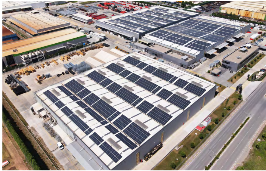
The photovoltaic system in Sakarya, Turkey, covers the entire electricity requirements of this PERI production site.
